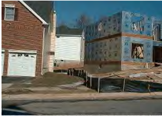
In sequenced construction, sites are completed in stages and completed portions are permanently stabilized before other areas are disturbed
